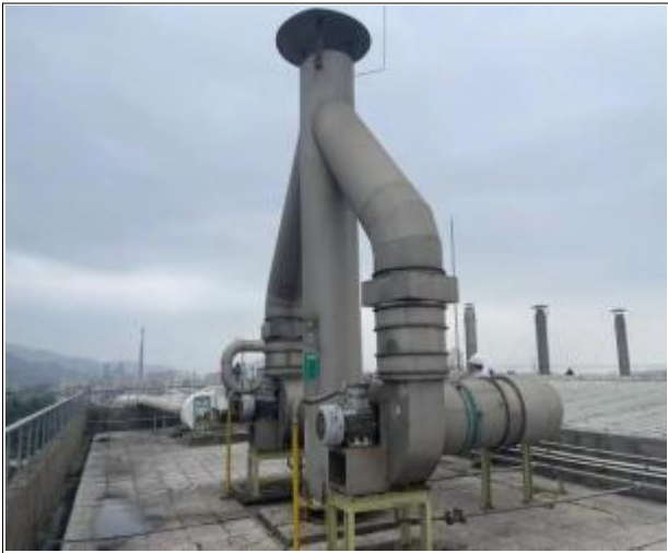
SM1 车间排气筒 (FQ-223-3)
